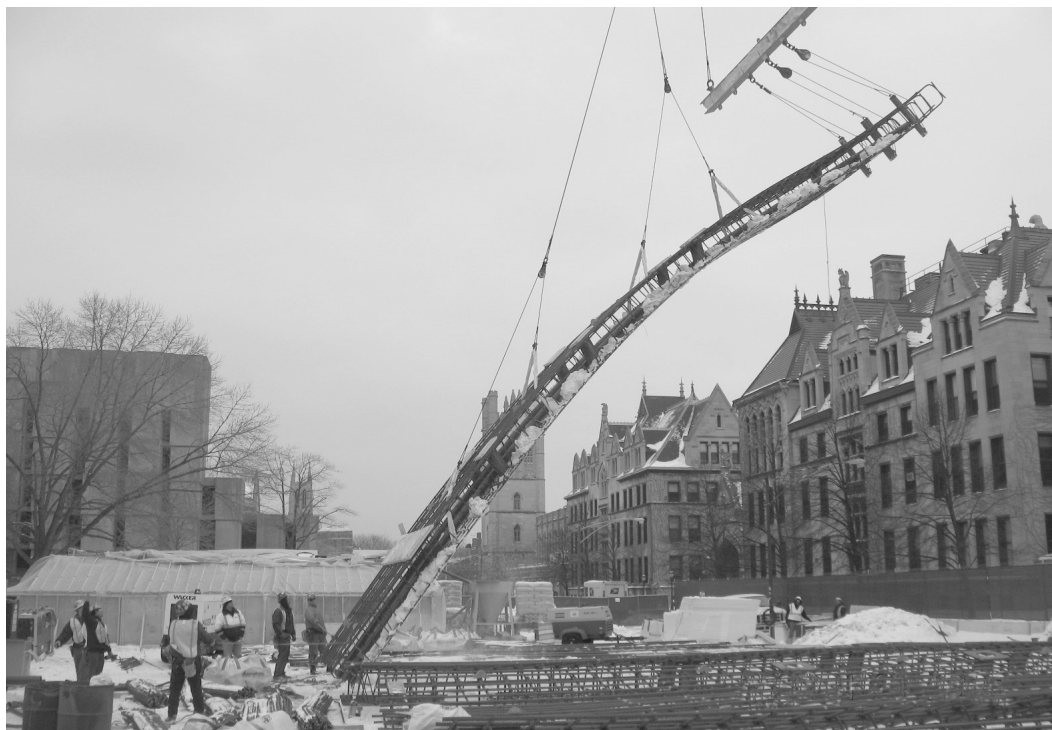
A crane lifts a 60-foot-long rebar cage that now forms part of the Mansueto Library's foundation wall. (Photo courtesy of Barton Malow)
