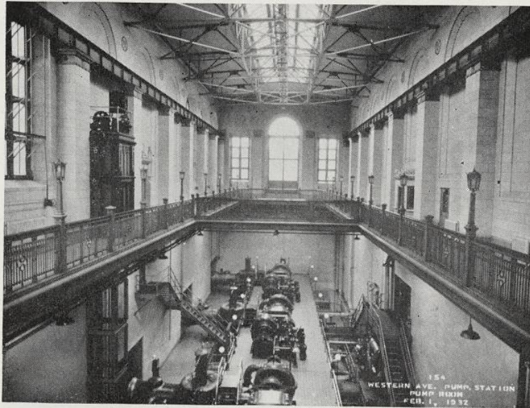
Figure 14—75 M.G.D. Turbine driven Centrifugal pumps—Western Avenue Station
